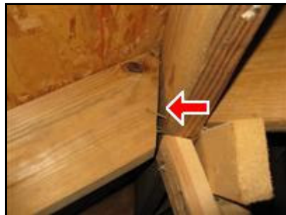
D. Picture 5 Left front of home
