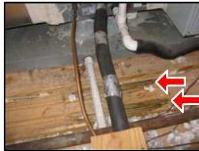
B. Picture 3 Black insulation needs repair
