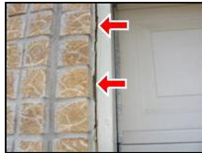
E. Picture 21 Gap between brickwork
