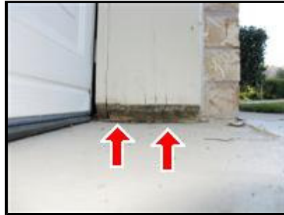
E. Picture 11 Garage trim needs sealing
