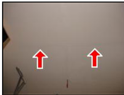
F. Picture 1 Slight water staining
