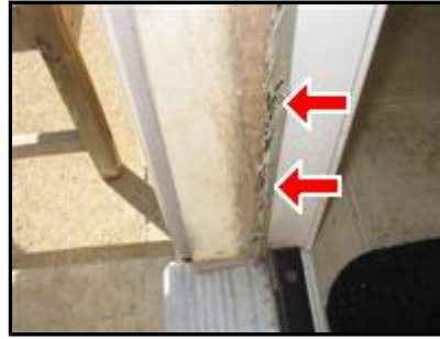
G. Picture 1 Damaged weatherstripping
