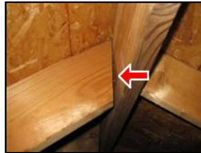
D. Picture 4 Left front rafter gap
