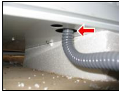
A. Picture 1 Furnace gas pipe
